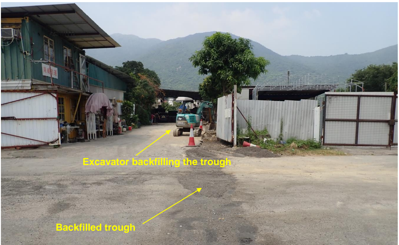
Photo 4 showing an excavator possibly backfilling at one end of the trough inside the suspected illegal open storage in Shek Lau Po on 14 th Sep, 2018.
