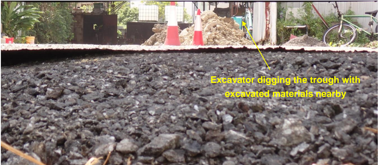
Photo 3 showing an excavator digging at one end of the burrow inside the suspected illegal open storage in Shek Lau Po on 13 th Sep, 2018.
